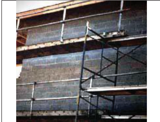
This scaffold is not in compliance with the regulations because it mixes several different scaffold components in the same scaffold. The guardrails are also improper because they are not complete.
