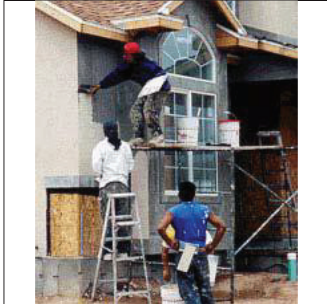
These workers are not protected from being struck by falling objects because they are working around/under other workers and not wearing hardhats.
